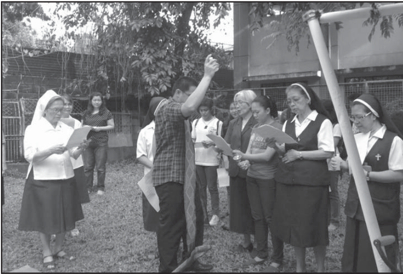
Sisters in Quezon City gather for the ground breaking of the new addition to the Sisters of Mount Carmel Catholic School. The Philippine government has added two years to the high school curriculum. Additional classrooms were needed to fulfill the mandate. The groundbreaking was August 23.
